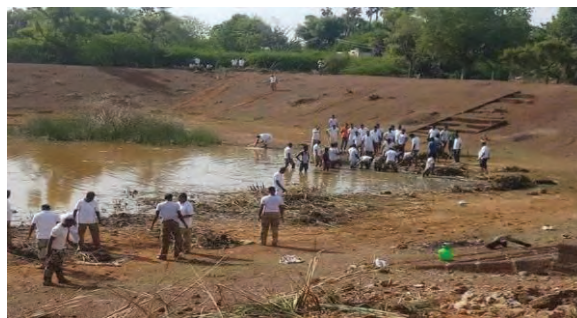
Jal Shakti Abhiyan; Restoration of Ponds by ESMs at ZSBO in August 2019
